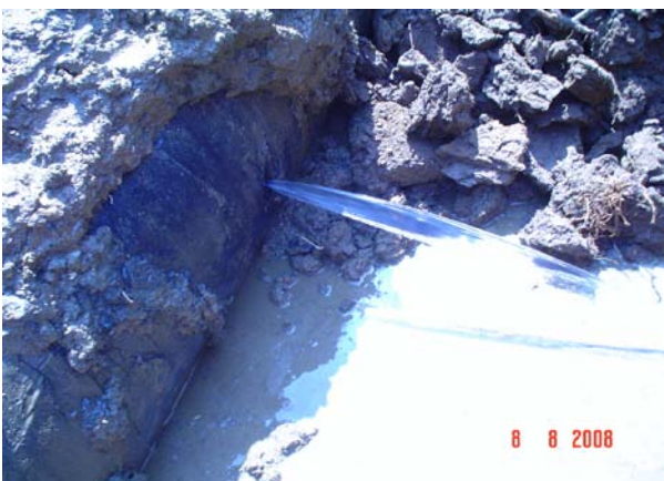
Picture 7 Water leakage from the steel pipes
