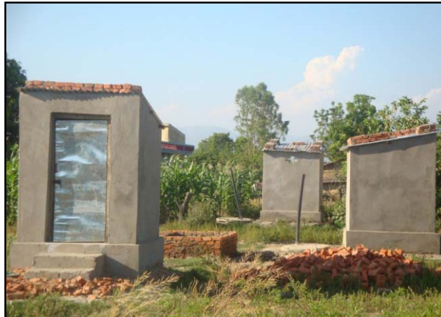
Fig. 4 HH latrine constructed through OBA in Shibnagar TP. Source: Nepal: Second Small Towns Water Supply and Sanitation Sector Project
